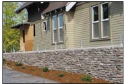
Special thanks to Bruce Fortner and Tom Godwin for completion of the stone work on our wheelchair ramp entrance.
